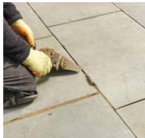
6. Prepare a damp mortar mix of 1 part cement to 4 parts building sand for jointing, pressing firmly onto the joints to produce a dense, impervious surface that will drain water across the paving to your drainage solution.
