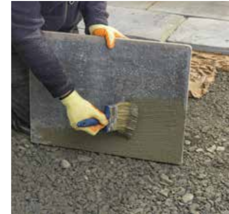
3. Paste to the rear of the paving a slurry backing prior to laying.
