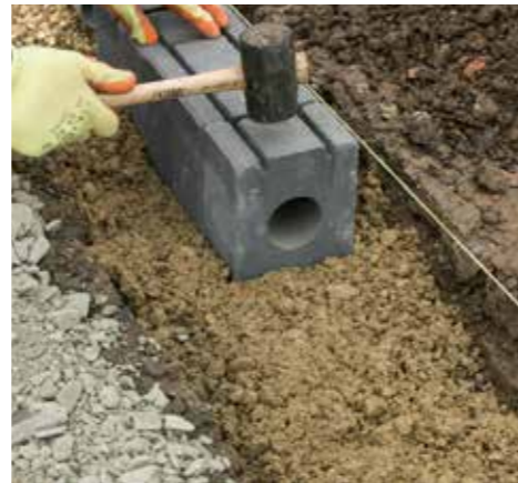
4. Lay the units onto a freshly mixed workable bedding concrete making sure you achieve a tight connection between each unit.
