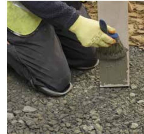
3. Paste to the rear of the paving a slurry backing prior to laying.
