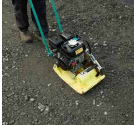
1. Prepare the ground as normal with compacted hardcore, achieving the correct falls for drainage.
