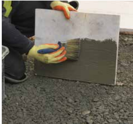
3. Paste to the rear of the paving a slurry backing prior to laying.
