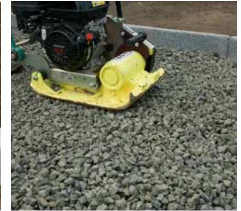
2. Prepare the ground with 100mm of 20mm clean crushed stone with well defined edges.
