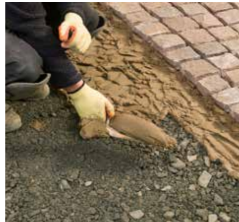
4. Prepare a full bed of mortar ahead of each pavior approximately 30/50mm thick.
