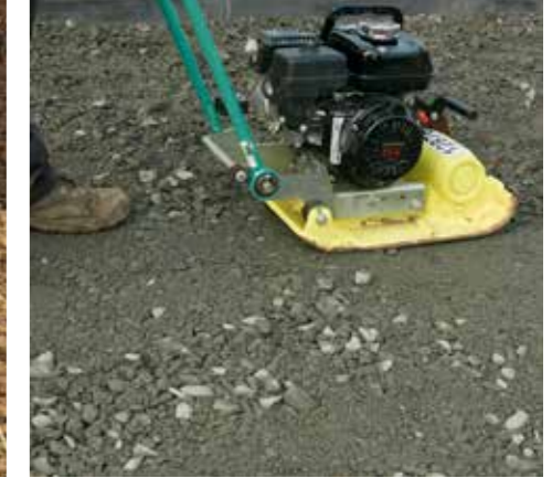
2. Prepare the ground as normal with compacted hardcore, achieving the correct falls for drainage
