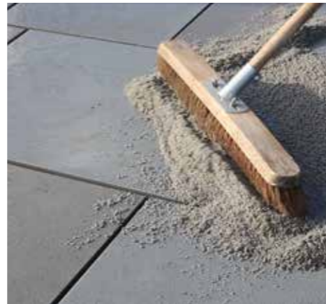
4. The material is brushed into the joints ensuring the joint voids are full
