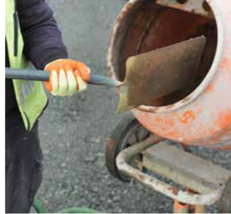
2. Mix a wet mortar mix of 1 part cement to 5 parts building sand.
