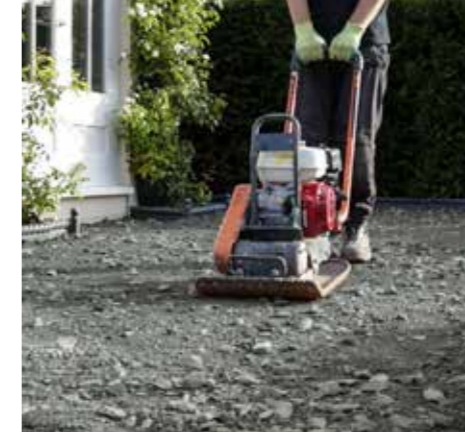
1. Prepare the ground as normal with compacted hardcore, achieving the correct falls for drainage.
