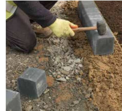
1. Install your choice of edge restraint on a concrete footing around the perimeter of the driveway.
