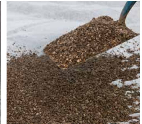
4. Prepare your laying course with 20mm of 6mm clean crushed stone. No need for compaction.
