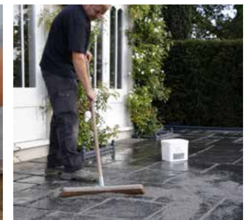
6. Brush in Stonemarket Fast Point jointing compound following the instructions on the tub, using plenty of water.
