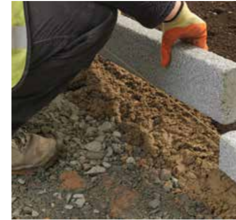
1. Install your choice of edge restraint on a concrete footing around the perimeter of the driveway.
