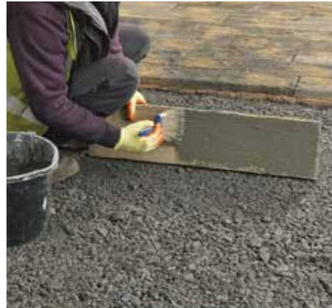
3. Paste to the rear of the paving a slurry backing prior to laying.
