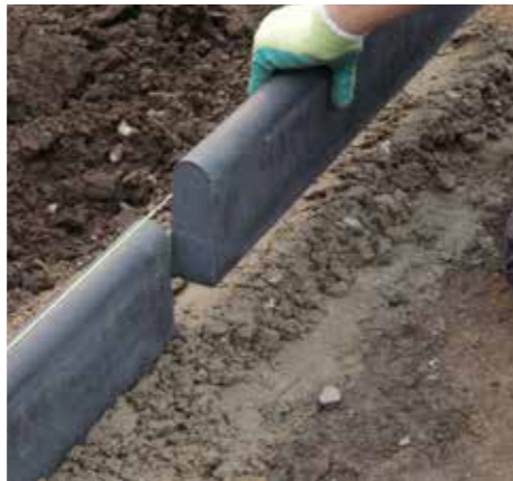
1. Install your choice of edge restraint on a concrete footing around the perimeter of the driveway
