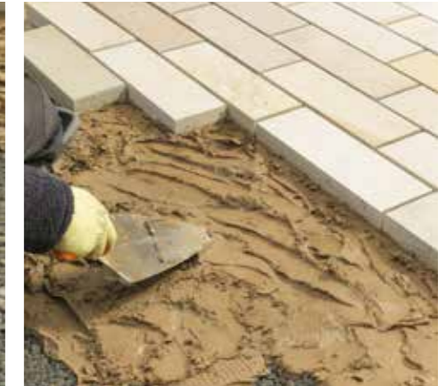
4. Prepare a full bed of mortar ahead of each flag approximately 30/40mm thick.
