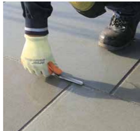
6. The joints are struck off using a pointing iron. Any gaps that are revealed are refilled with Fast Point.
