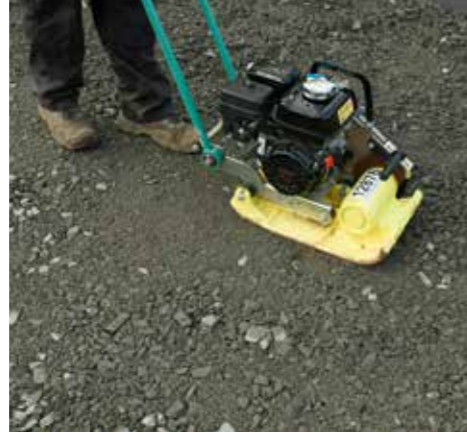
1. Prepare the ground as normal with compacted hardcore, achieving the correct falls for drainage.
