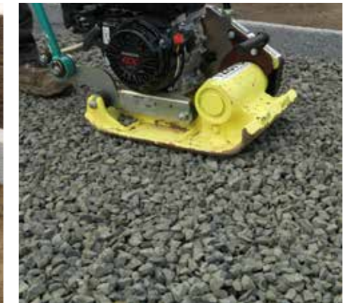
2. Prepare the ground with 200mm of 20mm clean crushed stone with well defined edges.
