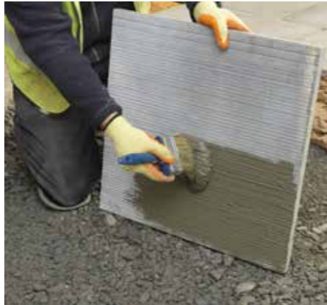
3. Paste to the rear of the paving a slurry backing prior to laying.
