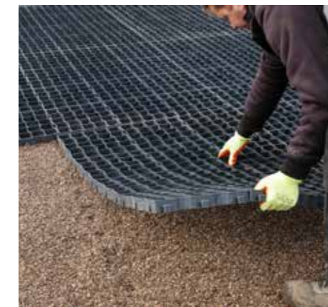
5. Install your grid ensuring the edge is 5mm from the edge restraint to allow for expansion.
