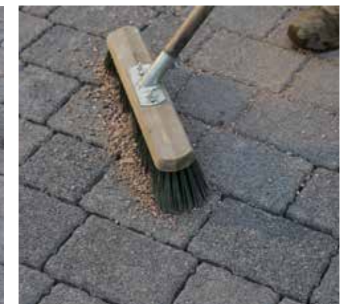
6. Fill the joints with 6mm clean crushed stone, using a stiff brush.
