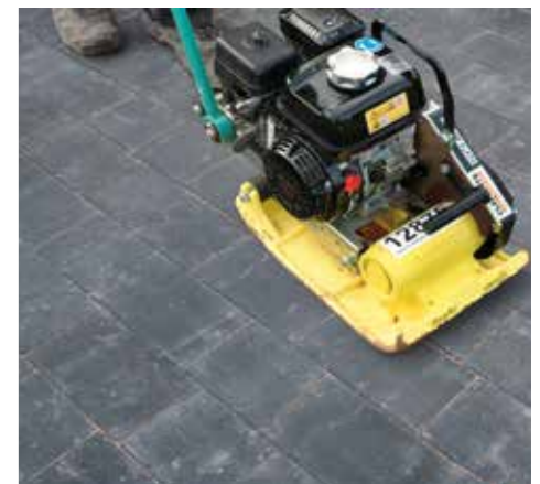
6. Using a plate vibrator compact the blocks and refill hungry joints with kiln dried sand.
