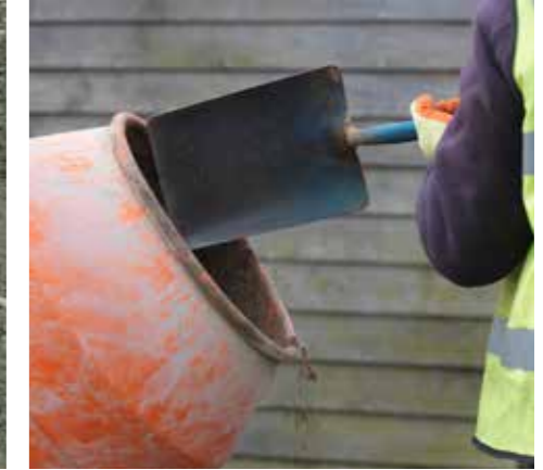
2. Mix a wet mortar mix of 1 part cement to 5 parts building sand.
