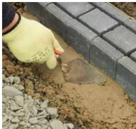
5. Haunch the units using bedding concrete of an appropriate thickness and depth.
