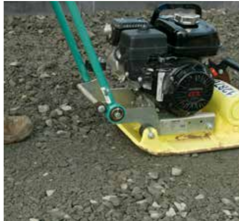
1. Prepare the sub-base in two layers of compacted 75mm MOT type 1 hardcore achieving the correct falls for drainage*.
