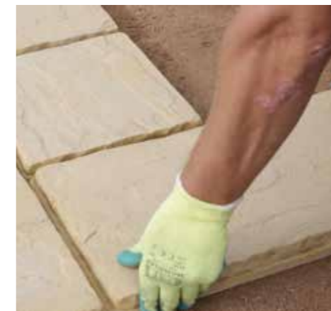
5. Make a solid connection when laying the NEXTpave to ensure a perfect uniform joint.
