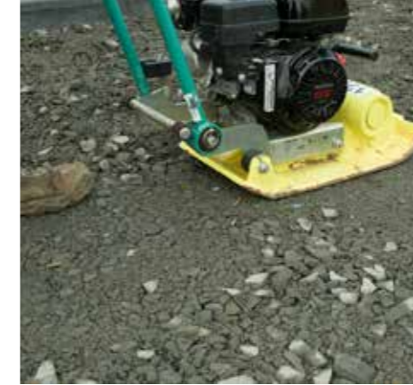
1. Prepare the ground as normal with compacted hardcore, achieving the correct falls for drainage.
