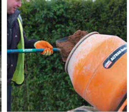
2. Mix a wet mortar mix of 1 part cement to 5 parts building sand.
