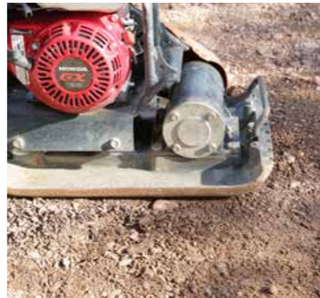
2. Prepare the sub-base in two layers of compacted 75mm MOT type 1 hardcore, achieving the correct falls for drainage*
