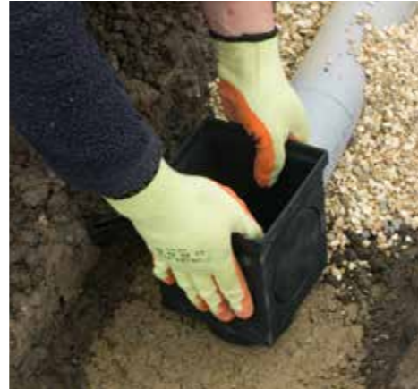
2. Drainar Outfalls and Rodding boxes should be installed first along with relevant pipe work to relevant soakaway or SuDs compliant system.
