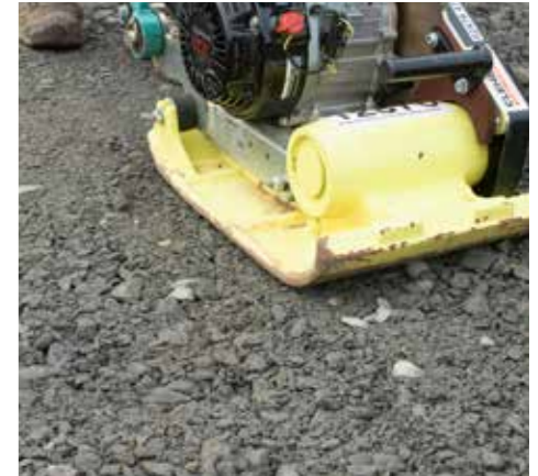
2. Prepare the sub-base in two layers of compacted 75mm MOT type 1 hardcore, achieving the correct falls for drainage*.
