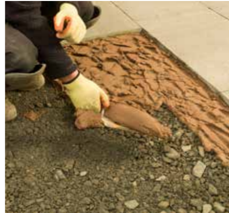
4. Prepare a full bed of mortar ahead of each flag approximately 30/40mm thick.
