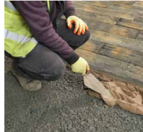
4. Prepare a full bed of mortar ahead of each flag approximately 30/40mm thick.
