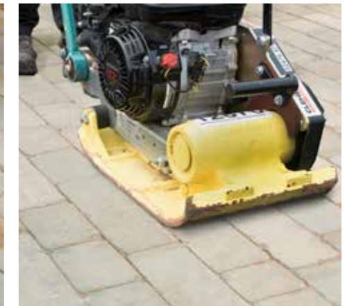
6. Using a plate vibrator compact the blocks and refill hungry joints with kiln dried sand.
