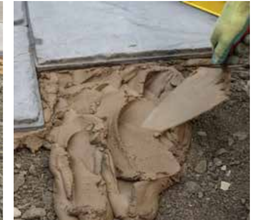
4. Prepare a full bed of mortar ahead of each flag approximately 30/40mm thick.
