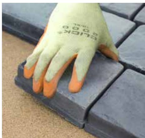
5. Make a solid connection when laying the blocks to ensure a perfect uniform joint
