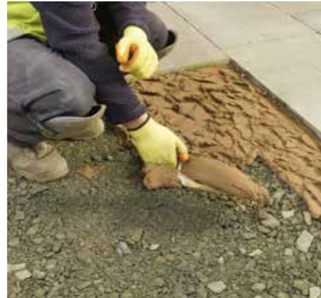
4. Prepare a full bed of mortar ahead of each flag approximately 30/40mm thick.
