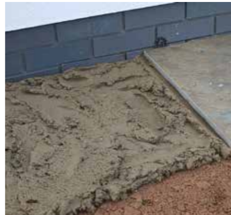
4. Prepare a full bed of mortar ahead of each flag approximately 30/40mm thick.
