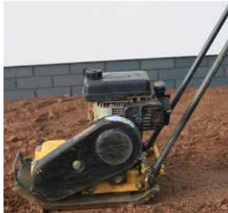
1. Prepare the ground as normal with compacted hardcore, achieving the correct falls for drainage.
