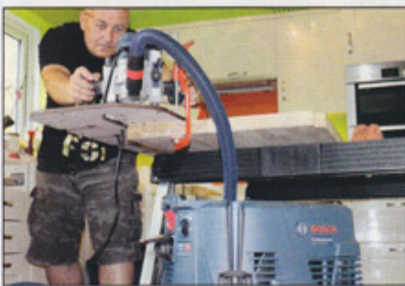
Take several passes to ensure a clean cut. Then reverse the worktop and make the mating cut
